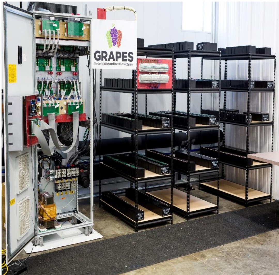
Medium Voltage Cabinet Level Prototype
