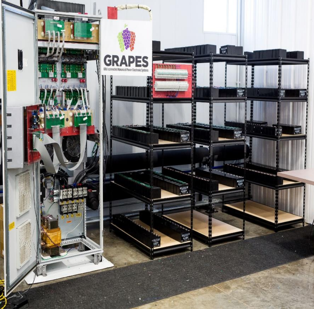
Medium Voltage Cabinet Level Prototype
